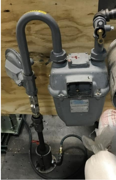
Figure 21: Utility 7 Meter Set (with Hook Pre-Fab Configuration)
