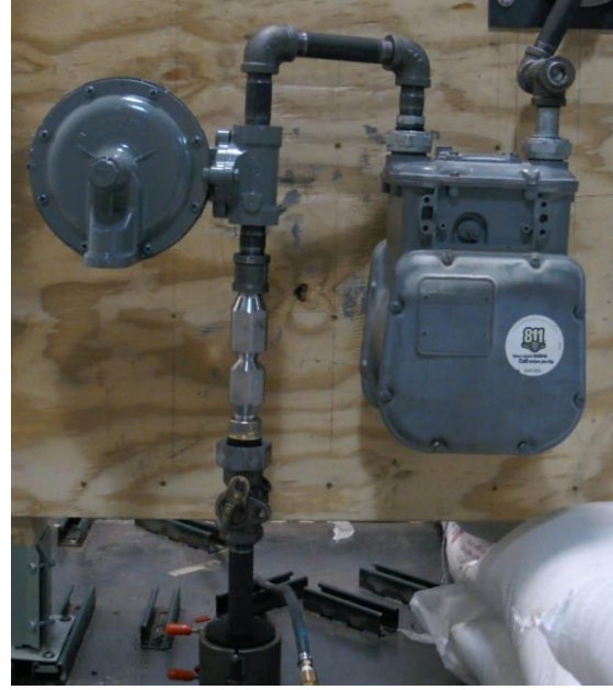
Figure 22: Utility 8 Meter Set (with Elbow Pre-Fab Configuration)
