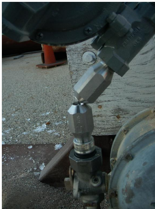
Figure 84: Close Up of Breakaway from Utility 1 Meter Set After First Drop Test
