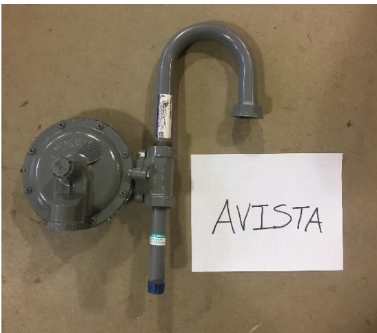
Figure 70: Utility 1 Meter Set
