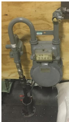
Figure 18: Utility 3 Meter Set (with Connector Bar)
