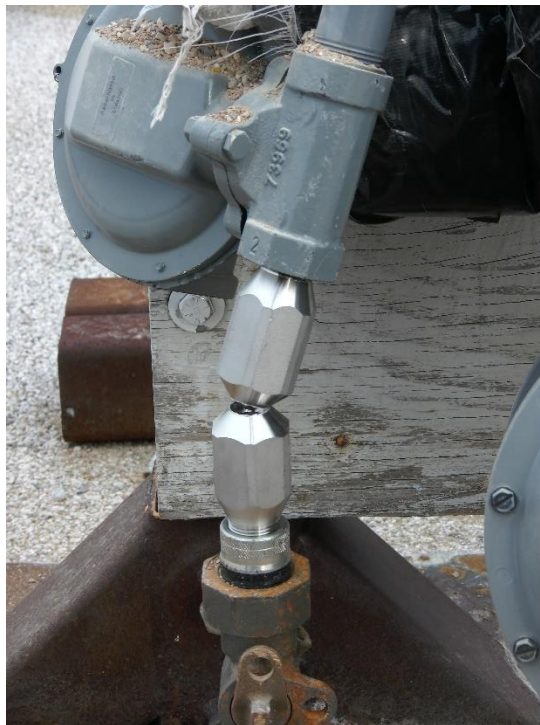
Figure 88: Close-Up of Breakaway from Questar Meter Set after Drop Test
