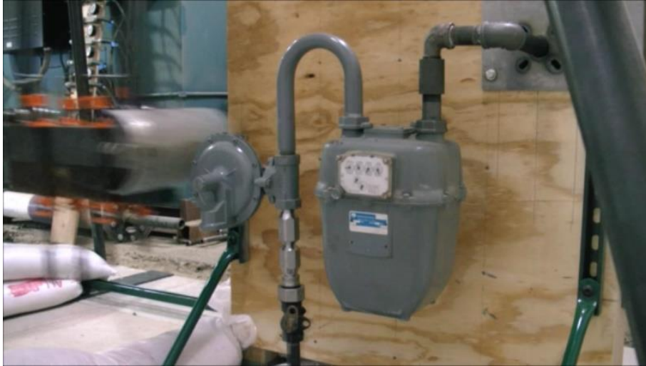
Figure 11: Impact Test on Utility 1 Meter Set with Breakaway and Regulator Left of Riser (Away from Meter) – Impacted Parallel to Wall from Regulator Side – Before Impact
