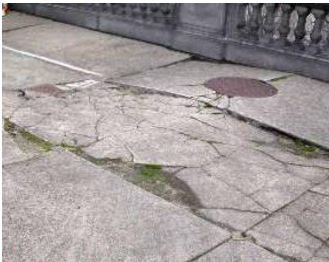
Frost heave formation at the pavement surface.
